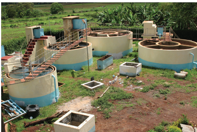
Fig 7.4 Water treatment plant in Rwanda
